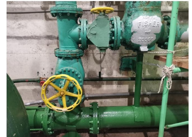
Pipes with potential biofouling
